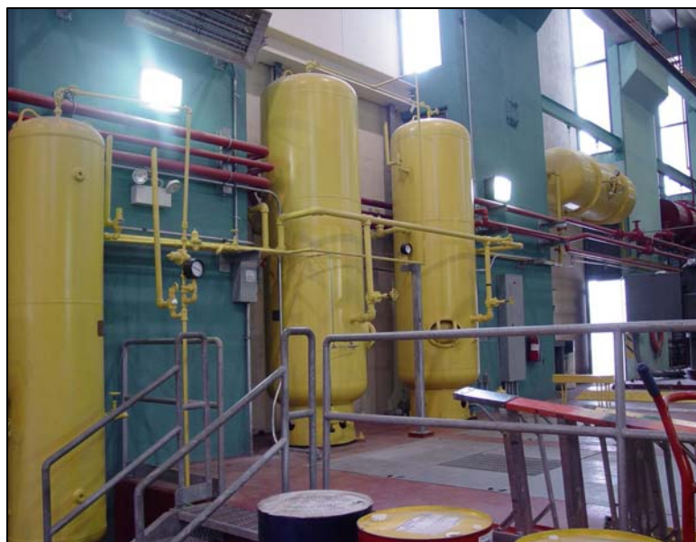
Air Suppression Interim Backflow Prevention System
