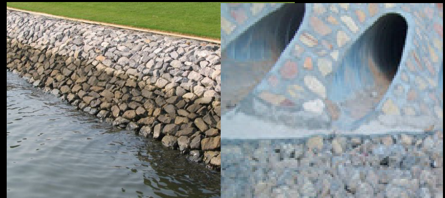
RIP RAP FOR SLOPE STABILIZATION AND MORE UNIFORM PIPE LENGTHS. CUT PIPES AT ANGLES TO CONFORM TO BANKS.
