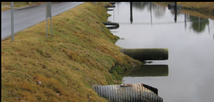
IRREGULAR EDGES AND PIPE LENGTHS
