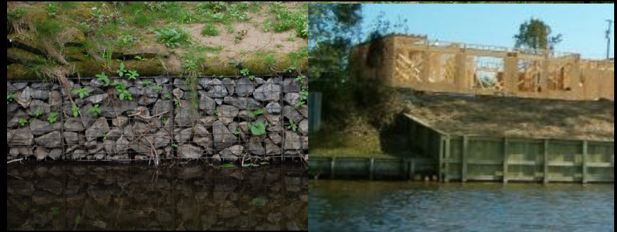
ROCK AND WIRE GABIONS OR PILING AND BULKHEAD TO CREATE SOLID EDGES AND STABLE SLOPES
