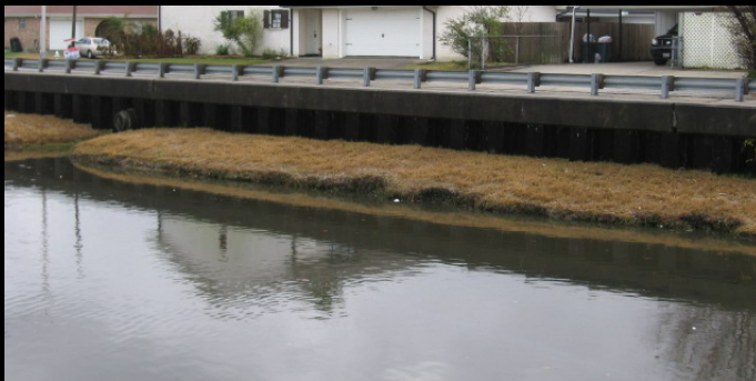
NO EMBANKMENT OR STEEP SLOPES
