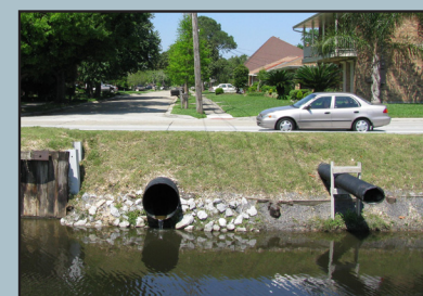
This photo of existing drain outfalls shows two completely different treatments. The pipe on the left is similar to how all outfall locations could be treated - trimmed back close to the bank, with gabion or rip rap underneath.
