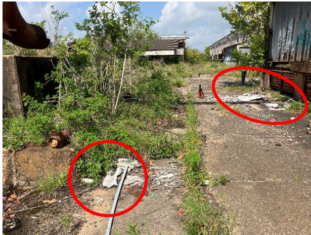
Photo of ACM building and construction debris.
