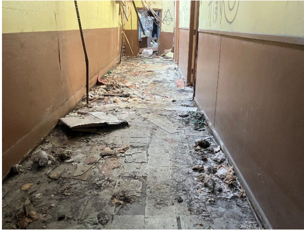
Photo of 9" x 9" Tan Floor Tile and associated Black Mastic sampled in Office Building.
