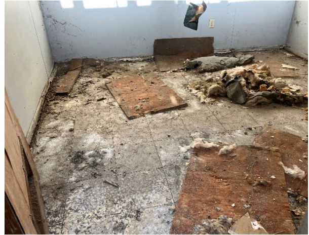
Photo of 12" x 12" Beige Floor Tile and associated Black Mastic sampled in Office Building.
