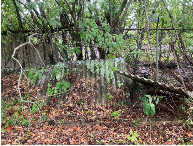
Photo of ACM building and construction debris.
