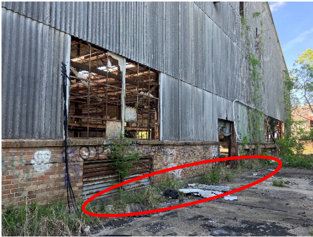
Photo of ACM building and construction debris.
