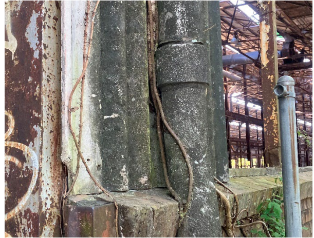
Photo of transite pipe and corrugated transite siding located on the exterior of the Factory Building.
