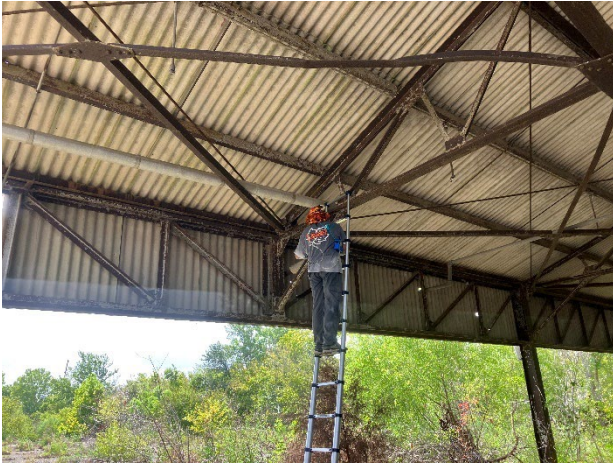
Photo of thermal system insulation pipe and corrugated transite roofing/siding for the Storage Structure.
