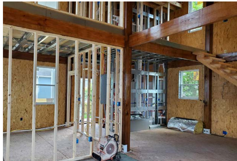
The recently updated Louisiana statewide building code is now one of the most stringent codes in the country
